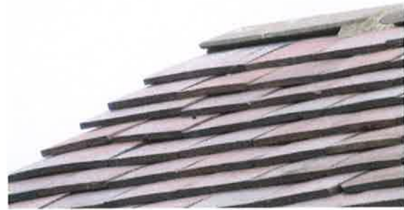
Gap at ridge tile.
